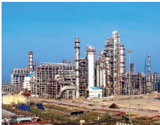
Grassroot unit of capacity 0.1 MMTPA at Guwahati Refinery
