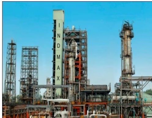
Grassroot unit of capacity 4.17 MMTPA at Paradip Refinery
