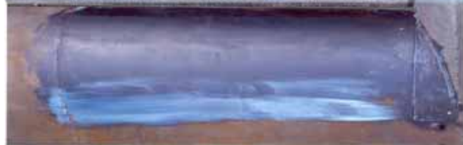
Method of applying Rust converter-First coat marine grade pyramid rust converter after cleaning by sand blasting:- Colour shade after application of rust converter (wide angle view) (1)
