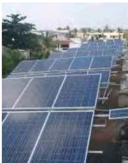
^ Solar photovoltaic water pumping systems
