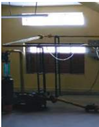
↗ Pneumatic transport of dry solids
