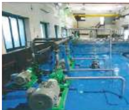
^ Facility developed for water metre evaluation
