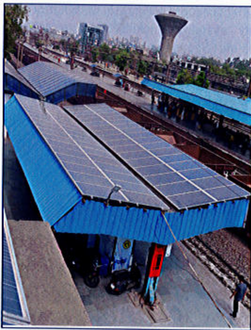
Fig. 17 Solar Railway Platform Shed Commissioned by CEL at Sahibabad Railway Station.
