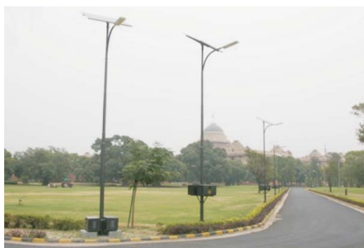
Fig 97: A view of Solar Street Lights installed by CEL at Rashtrapati Bhavan
