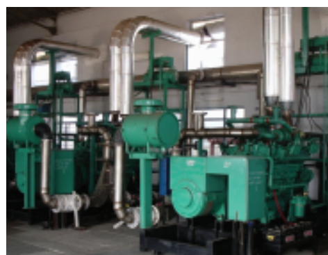
Gas Engines coupled to IISc Biomass Gasifier.
