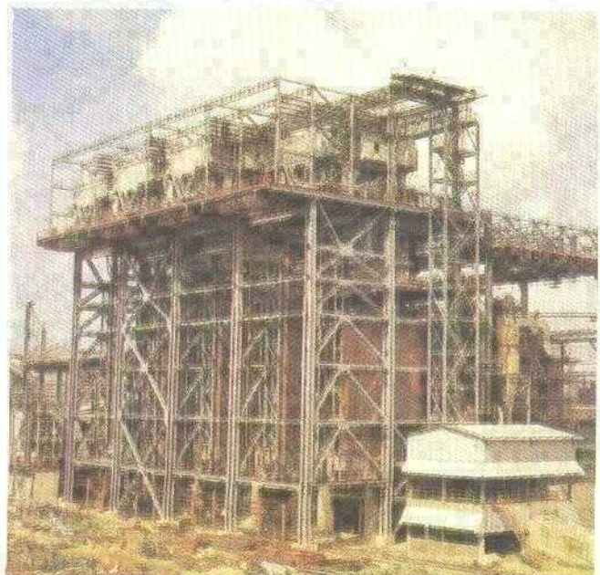
IX.2 Coke Dry cooling plant.
