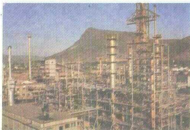
11.5 Plant for Ethylbenzene at Hindustan Polymers, Visakhapatnam.
