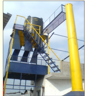
Methane Gas Collection Tower
