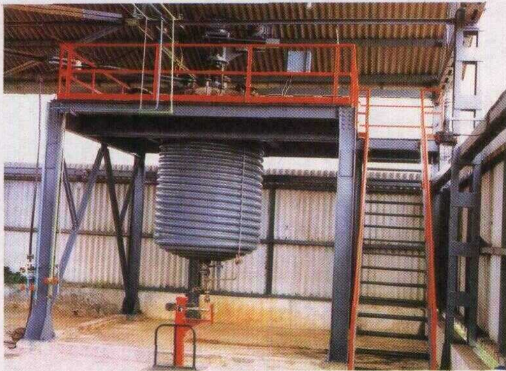
III.A.5 Catalyst Manufacturing unit
