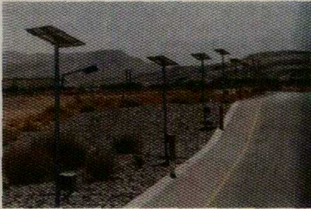
VIII.B.2 Solar Powered Street Lights supplied and installed by CEL at the Rusayl Industrial Estate (RIE), Oman.
