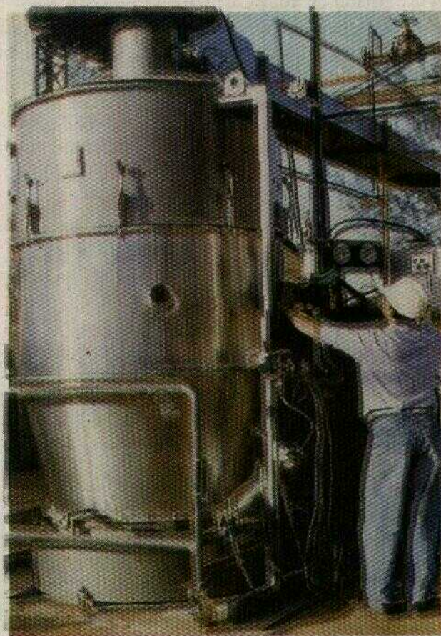
III.A.9 Equipment in Special Grade Alumina Pilot Plant
