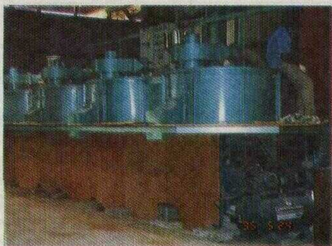
VII.A.6 Rice Husk Particle Board Plant at Malaysia
