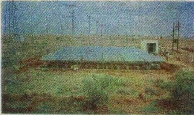
VII.B.1 15 KWp Grid Interactive SPV Power Plant installed by CEL in Kayathar Wind Farm (Tamilnadu).
