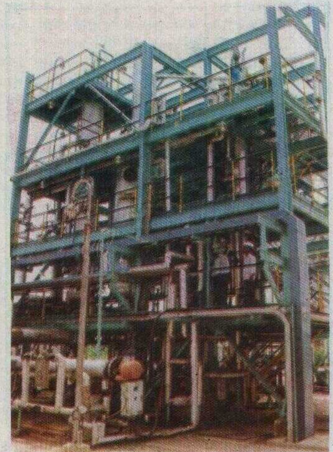
III.A.8. Rotating Disc Contactor Lube Extraction Pilot Plant
