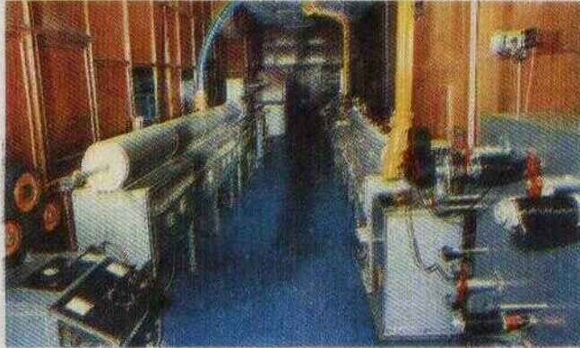
VII.A.4 Carbon Fibre Pilot Plant at NPL, New Delhi
