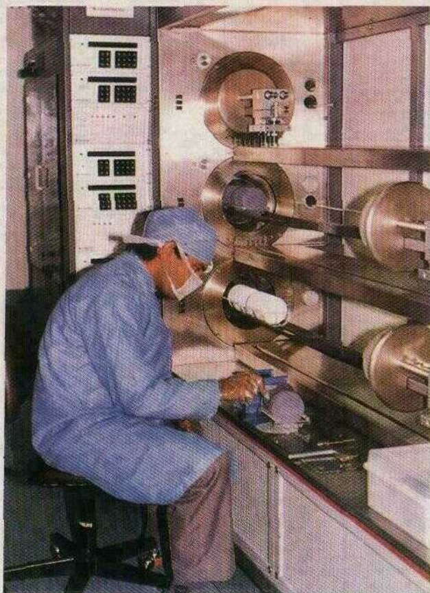
VII.B.4. Diffusion furnace with automatic loading/unloading and gas controlled facility at the SPV plant at CEL
