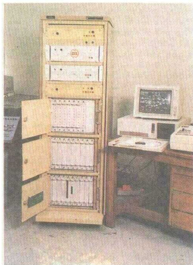
VII B.3 Solid State Interlocking System Under Development for Railways
