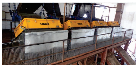
50 - 13 mm modules at GMDC Lignite Beneficiation Plant
