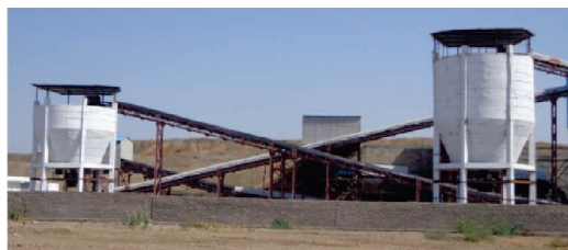
Overview of Lignite Beneficiation plant designed, erected, installed and commissioned by Ardee
