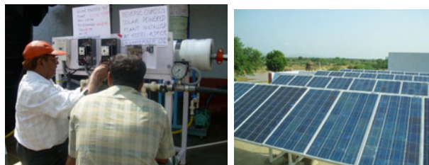
First solar power operated community scale reverse osmosis desalination plant installed in the country
