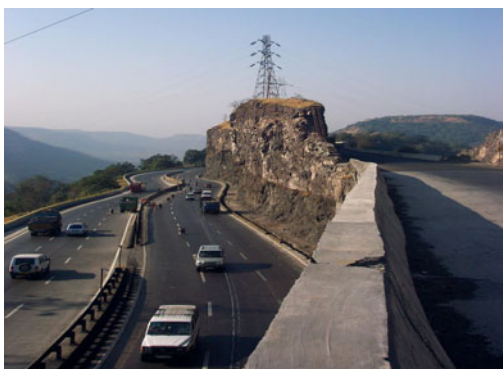
Landslide and Rockfall Site o Mumbai-Pune Expressway
