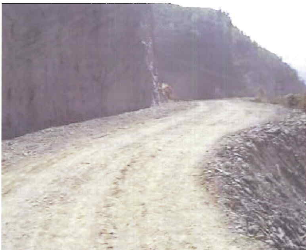
Fig. 36: View of final road after widening by controlled blasting (Midumkham Area), Mizoram
