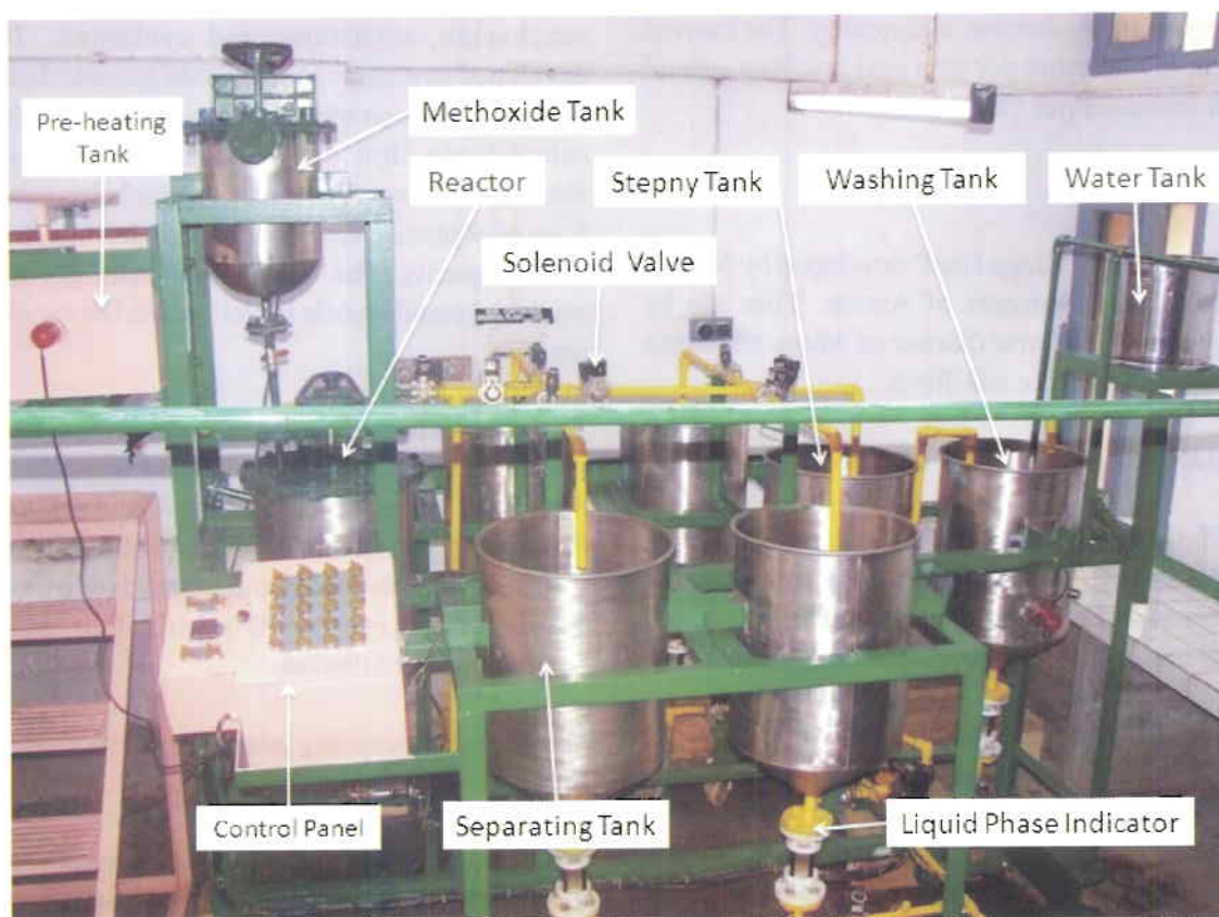
Fig.29: A view of the Bio-diesel plant
