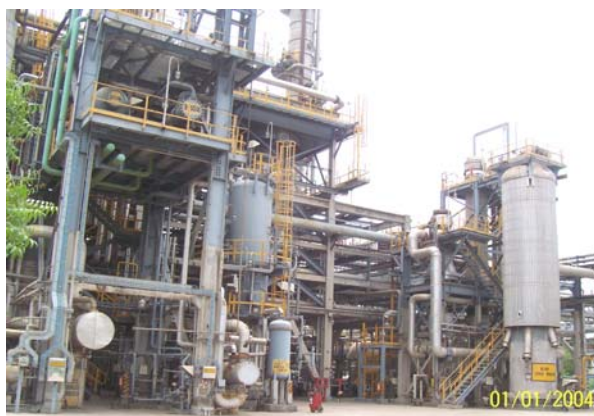
2500 MTA PDR Plant at RII Hazira
