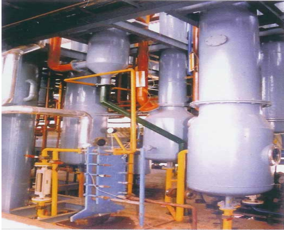
Vent Air Purification System
