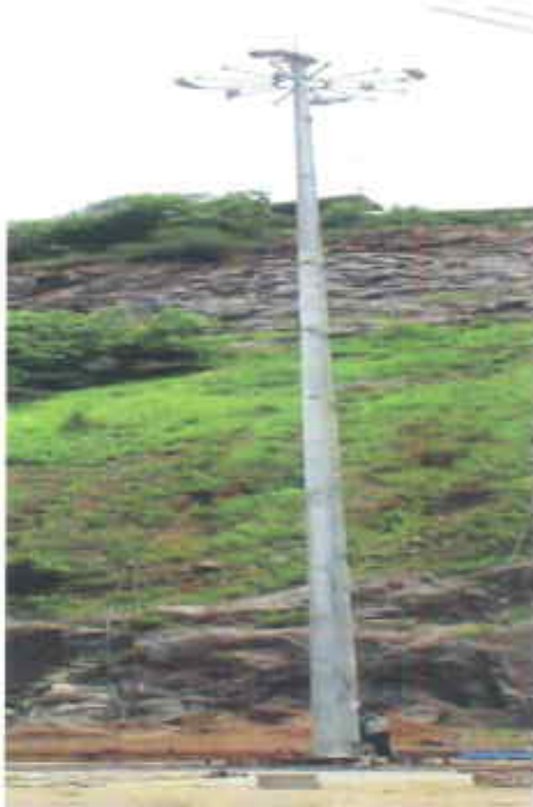
Fig. 1.46b. Bajaj Lighting Pole
