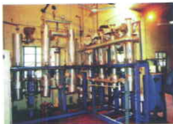
Fig. 1.19. Methanol Reforming Plant
