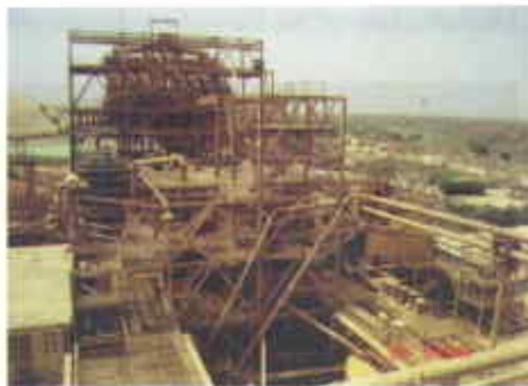
Fig. 1.70. 1000 tph phosphate ore beneficiation plant at Talba Mine, Senegal
