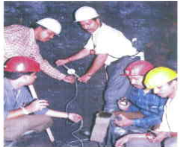
Fig. 1.36. Installation of a vibrating wire stress meter in a horizontally drilled hole
