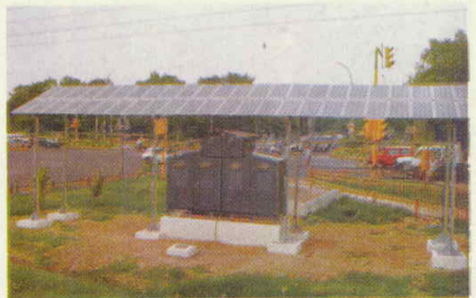
VIII.B.4 CEL's Solar PV powered Traffic signal lighting system - installed in New Delhi
