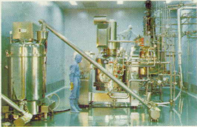
III.A.1 State-of-the-art 'Sterile' Bulk Manufacturing facility
